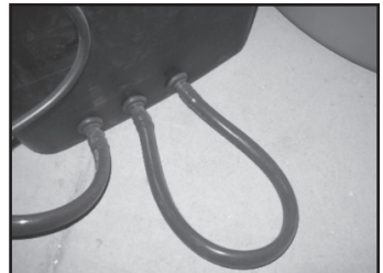
Unused outlets connected with tubing
